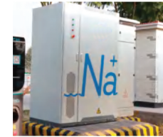
Hi resilience low volatility Sodium ESS solutions
